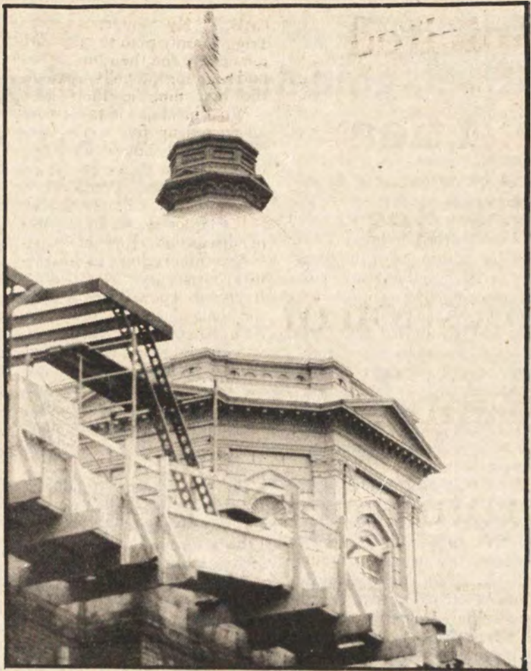
Construction on the new golden dome atop St. Ed's hall is progressing rapidly (photo by Chris Salvino).
